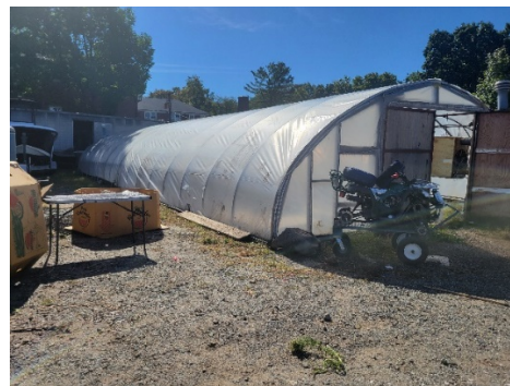
The condition of the exterior of the two greenhouses indicate issues caused by lack of maintenance. As seen above, junk and work equipment are strewn around haphazardly.
