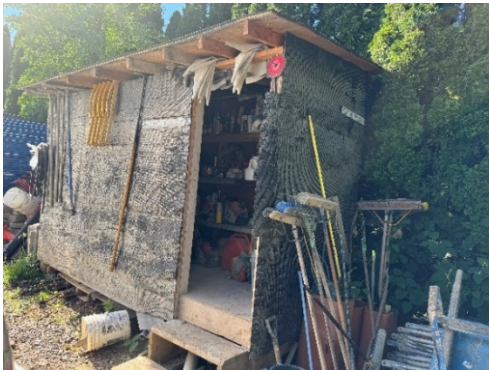
View of the dilapidated wooden storage shed to the rear of the greenhouse in the southwest corner of the property and the surrounding debris.
