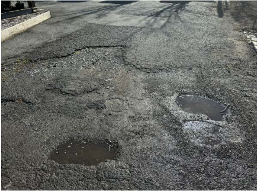
View of the parking lot, proximate to the glass paneled greenhouse, showing signs of decline with cracked pavement and potholes.
