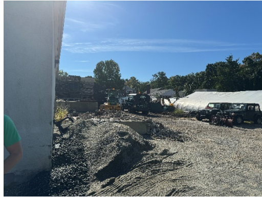
View to the rear of the five-door garage looking towards the greenhouses and the southeasterly portion of the rear property.
