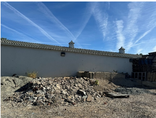
View looking towards the rear of the five-door garage. The site is strewn with debris.
