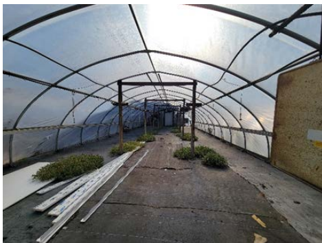
View of the interior of one of the green houses. There are large weeds growing through warped, make-shift plywood flooring. This indicates lack of maintenance.
